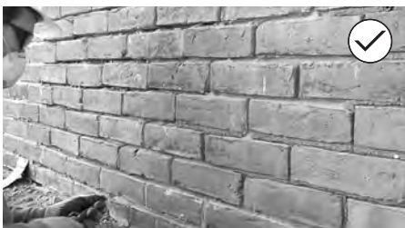
9. Re-point deteriorated masonry mortar joints.
